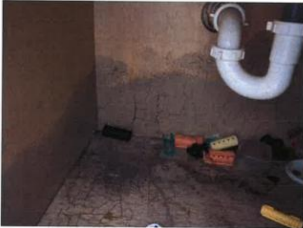
176. Building No. 19 – View of evidence of leak in 3840 McRee Avenue.
