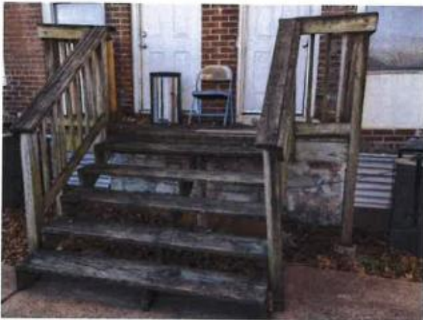
188. Building No. 21 – View of damaged wood stairs.
