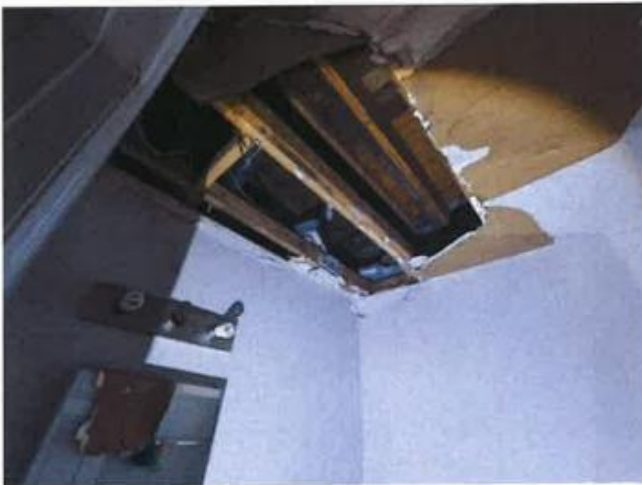
191. Building No. 22 – View of 3857 McRee Avenue ceiling with evidence of moisture intrusion.
