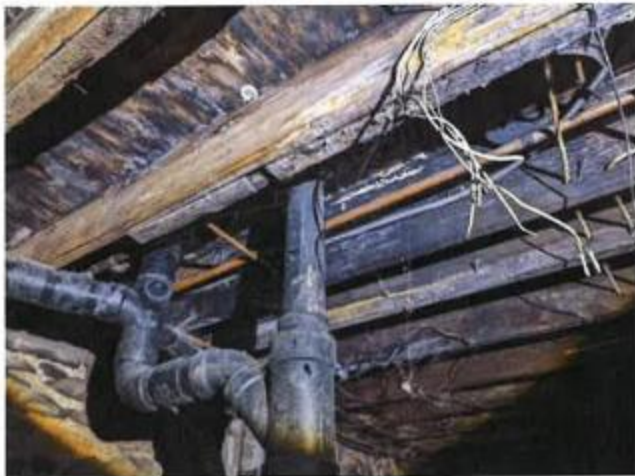
184. Building No. 20 – View of fire damaged wood joists and decking at 3844 McRee Avenue.
