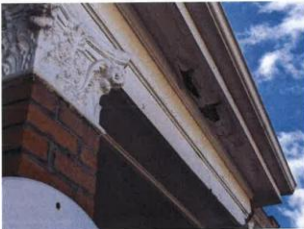
174. Building No. 19 – View of deteriorated soffit.
