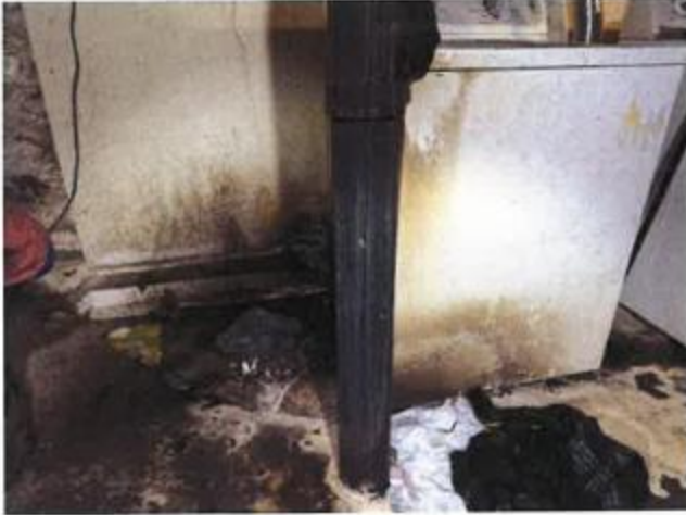
178. Building No. 19 – View of evidence of leak in 3840 McRee Avenue.
