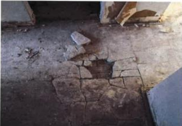
165. Building No. 17 – View of damaged concrete topping in 3825 McRee Avenue.
