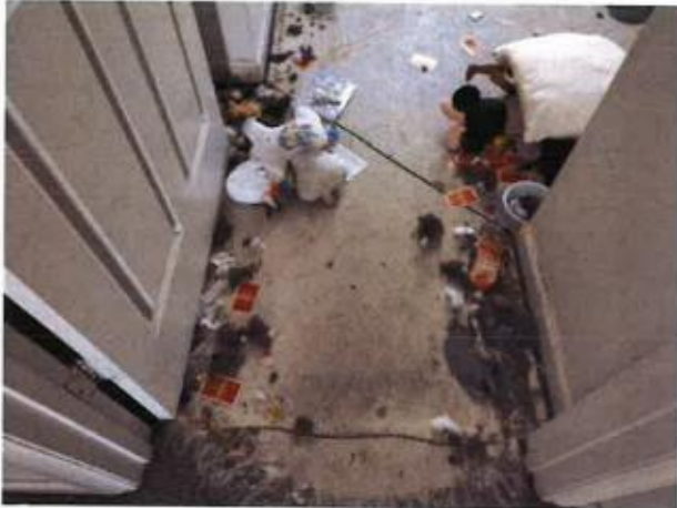
169. Building No. 18 – View of damaged flooring in 3837A McRee Avenue bedroom.
