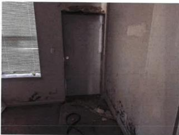
170. Building No. 18 – View of damaged finishes and door hardware, as well as organic growth in 3837A McRee Avenue.
