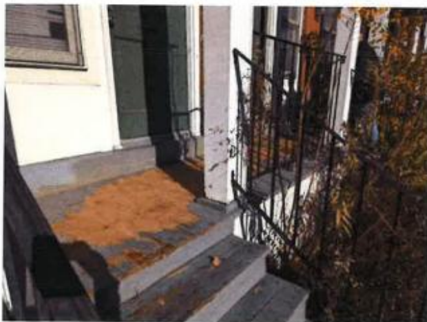
189. Building No. 21 – View of deteriorated paint at porch.
