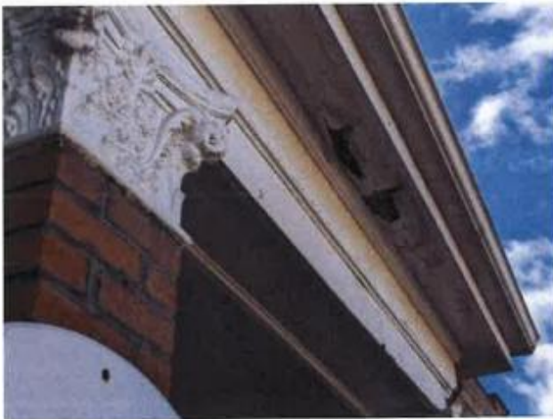
174. Building No. 19 – View of deteriorated soffit.
