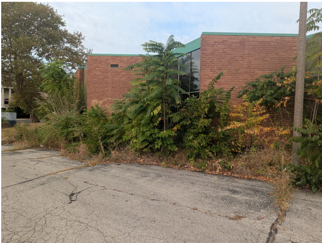
Eastern façade and uncontrolled vegetation
