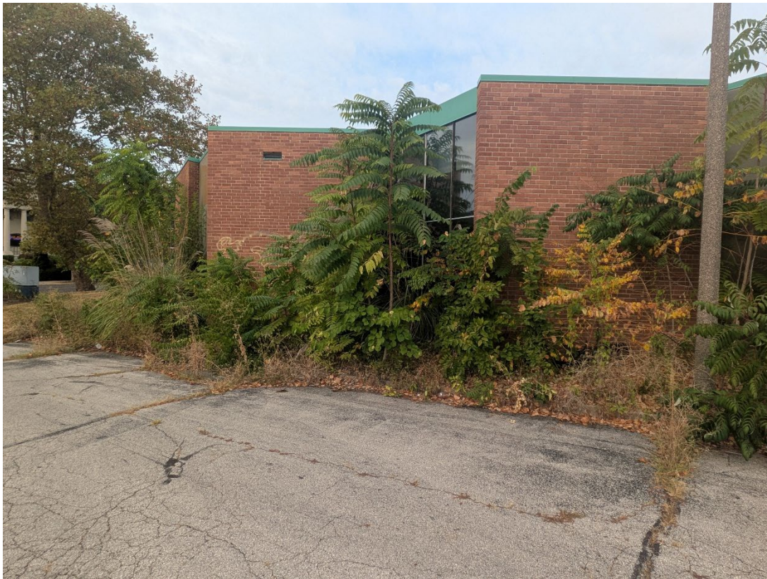
Eastern façade and uncontrolled vegetation
