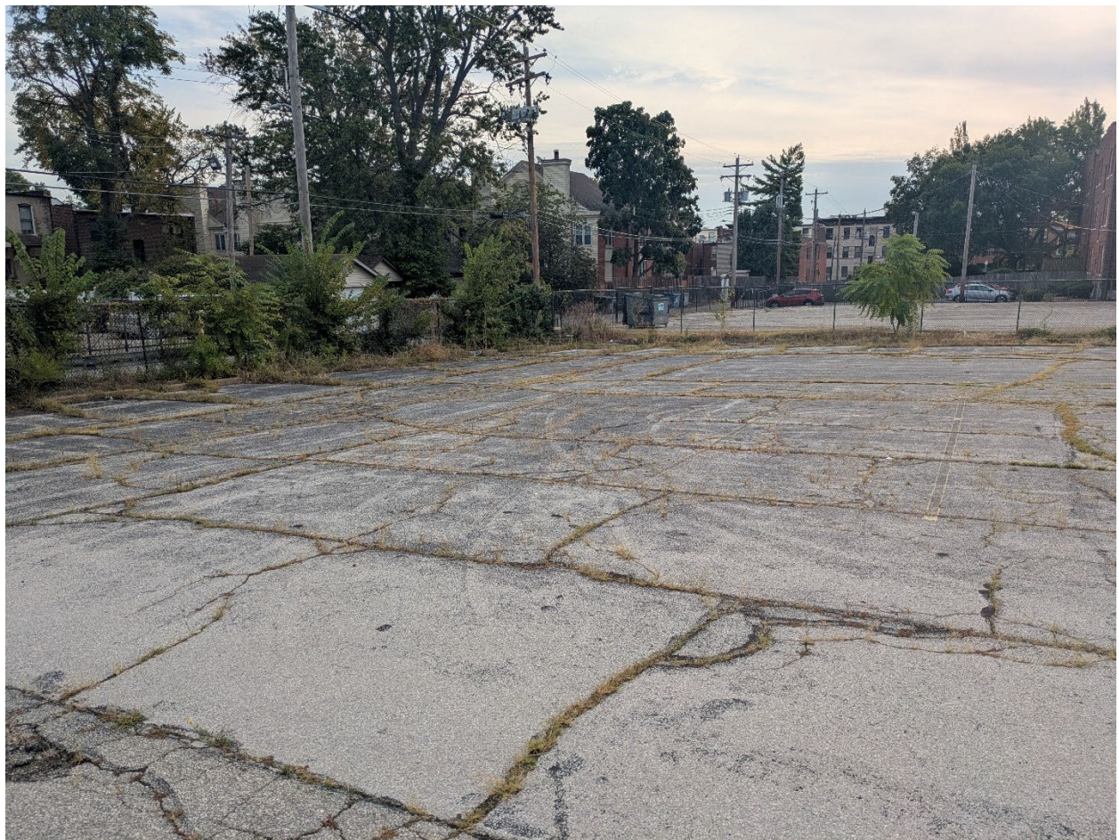
Figure 3 – Parking lot conditions.
