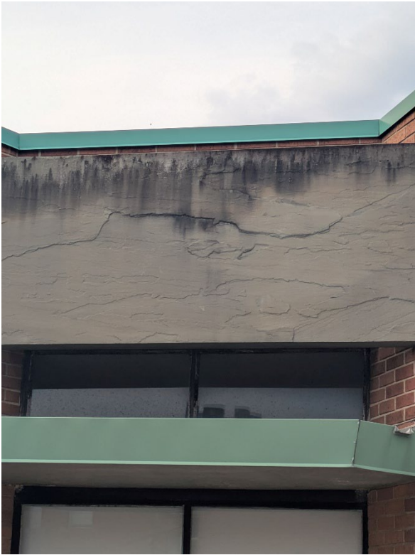
Figure 2 – Damage to exterior of building.
