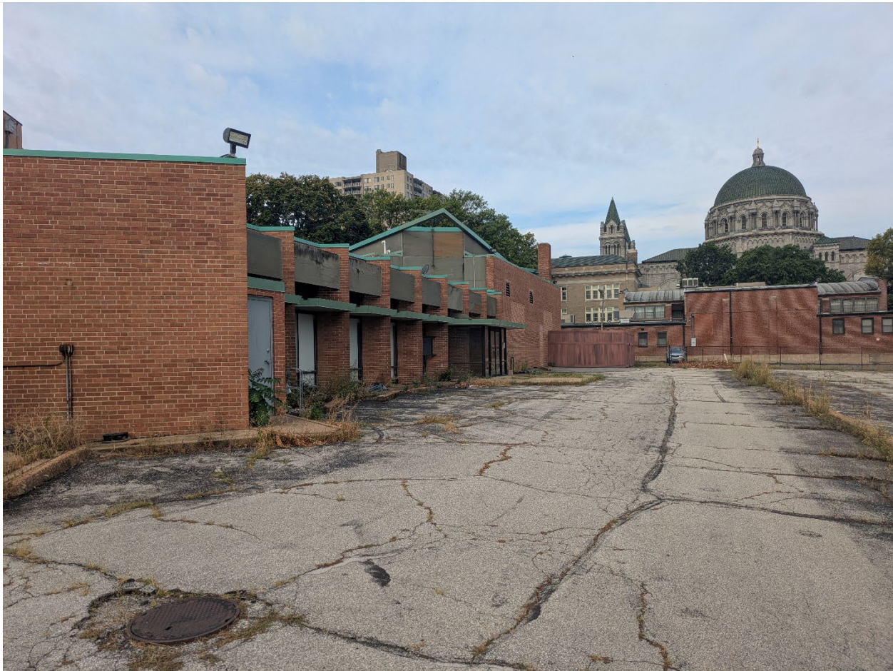
Figure 1 – North façade of the building and parking lot conditions.
